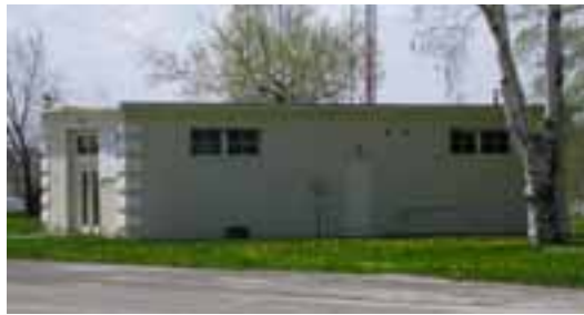
Unused 600-sq.ft. building that needs some roof work
